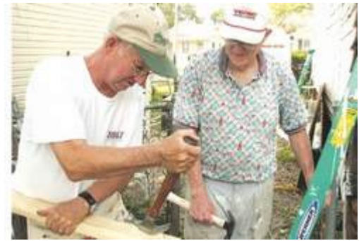
STAFF PHOTO | CECE NUNN Bill Harper (left) and Richard Younts, Wilmington Area Rebuilding Ministry volunteers, work recently on the at least 100-year-old house at 718 Wooster St. The ministry helps people with home repairs in New Hanover, Brunswick, Pender, Bladen and Columbus counties.
